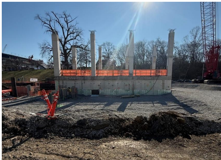
FIGURE 9: LOWER PUMP STATION SITE PHOTO
