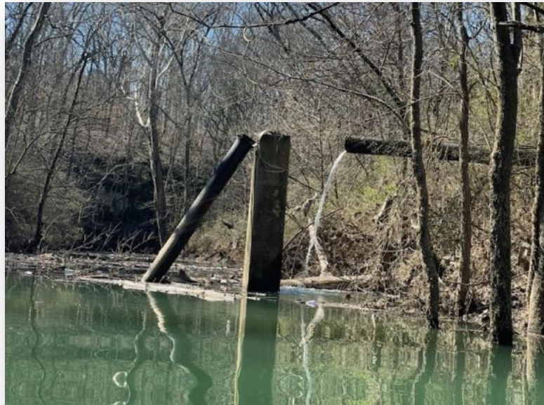
Photo of the Broken Aerial Sewer Line that was Repaired
